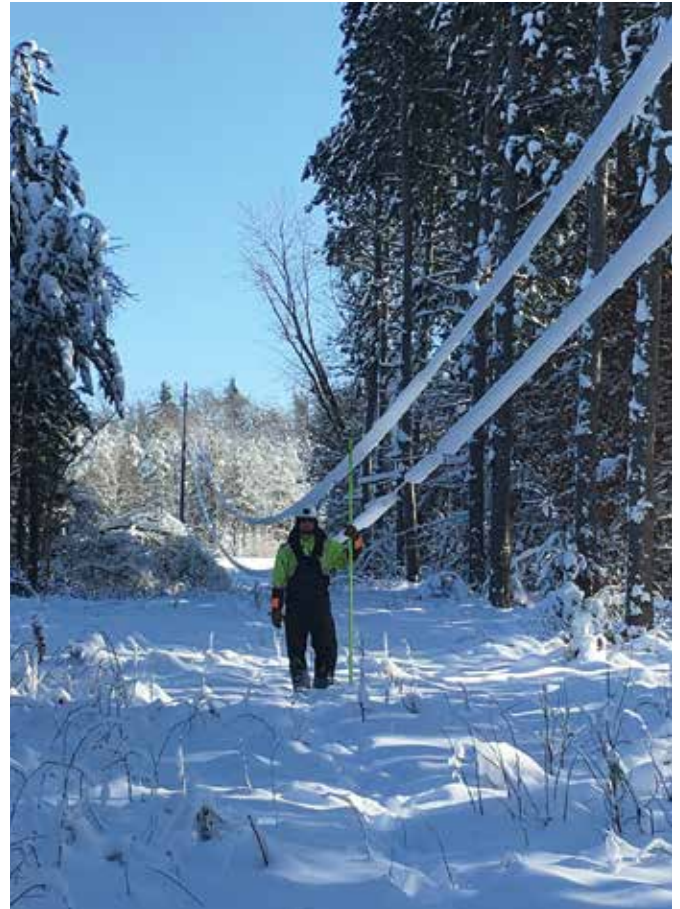
This photo, courtesy of Lineworker Alex G., shows the impact of heavy, wet snow on power lines.
