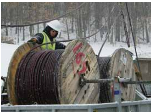
Left: Winter weather certainly does not deter necessary outside work for ECEC line workers. Despite the snow and extreme cold, Beau Blade and Terry Gilbertson (behind spools) continue to work laying out cable at Curt Manufacturing, a commercial and industrial co-op member, earlier this year.
