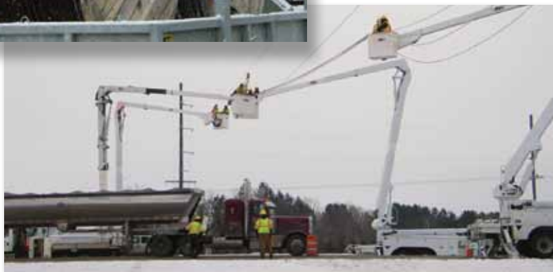
At one point six buckets, each with two-person crews from Eau Claire Energy Cooperative and Dairyland Power Cooperative, were up on the steel over Hwy 53 in Hallie. These crews pictured were stringing power lines across the highway to connect with the new East Hallie substation that will provide needed power for commercial growth in ECEC's service territory, including Lake Hallie, Seymour, and Lafayette. Communications was key since this project included 21 men and 11 bucket trucks.
