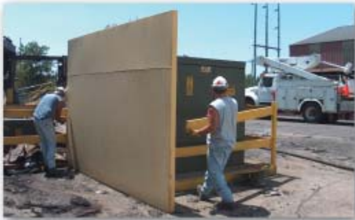
The steel wall to the left of the transformer helped to protect Eau Claire Energy Cooperative's electrical transformer from the severe heat of the fire. ECEC Line Workers Keith Kaufman and Rick LaPointe remove the protective barriers before inspecting the transformer and the switching enclosure. (Photos by Randy Baier and Line Worker Perry Gilbertson.)
